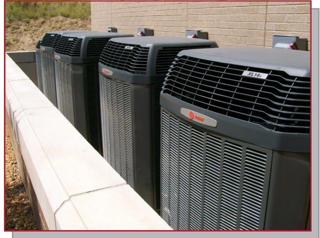
Bethel Middle School uses a variety of high efficiency Trane Systems like these 16-SEER XL16i condensing units to achieve reduced energy costs and consumption
